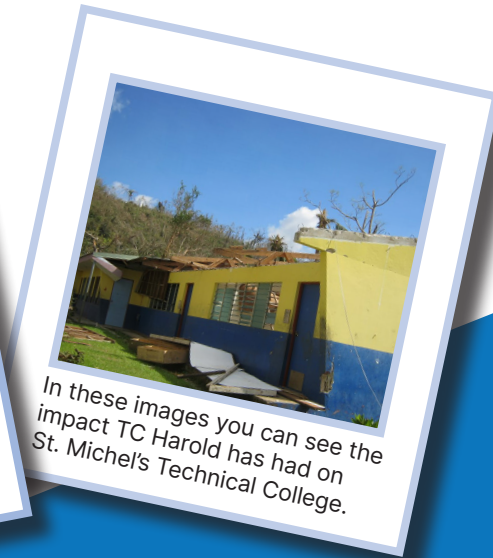
During Tropical Cyclone Harold, the roofs were ripped off homes.
